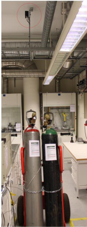
Figure 1 - Temporarily GC instalment with hydrogen detector (red ring)
