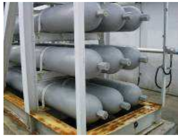
Figure 2. Cylinders at hydrogen station (Shut down inspection is conducted using a fiberscope)
