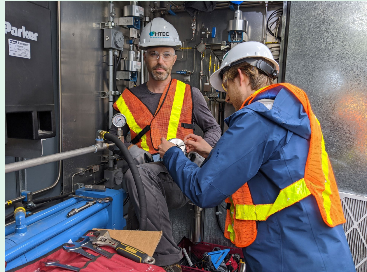
Hydrogen Compressor Maintenance
