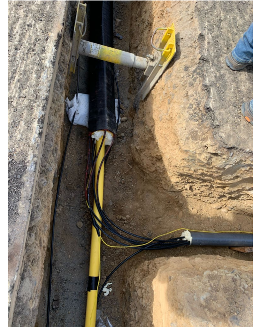
Fiber Optic Installation along a pipeline Photo Courtesy of Paulsson Inc (PI)
