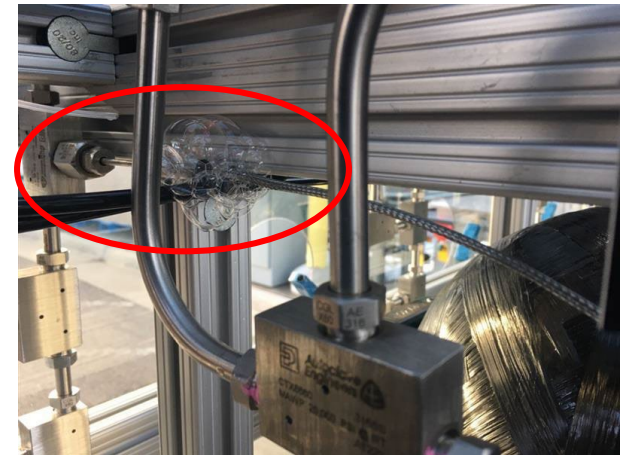
Small leak identified by a soap solution
