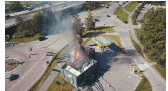
Hydrogen Refueling Station Explosion Norway, 2019
