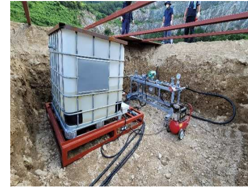
<Fuel tank and fuel supply system>
