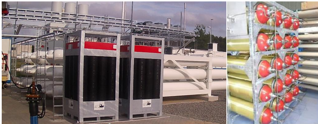
Figure 2. Buffers for hydrogen refuelling stations (vertical Type II cylinders and horizontal Type I tubes).
