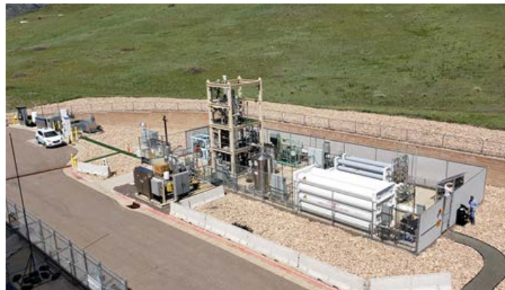
Figure 13: NREL’s Hydrogen Infrastructure Testing and Research Facility
