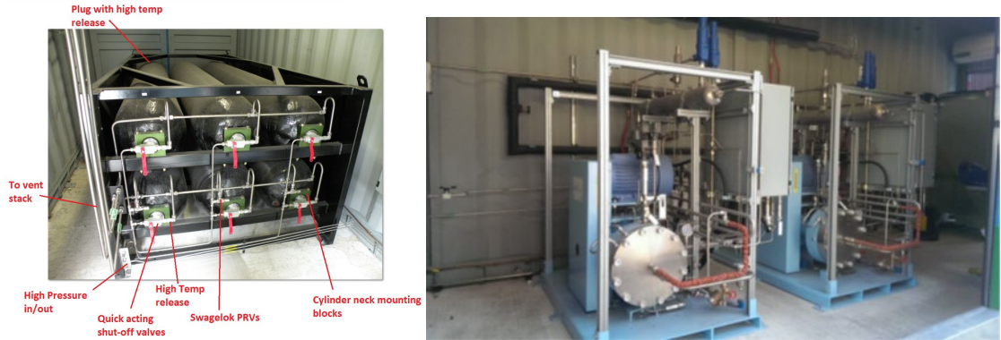
Figure 3. Key components of selected large enclosure (typical 40-ft container): HP H2 storage skid. Credit: Andrei V. Tchouvelev (ref. Canadian Tire Pilot Project).
