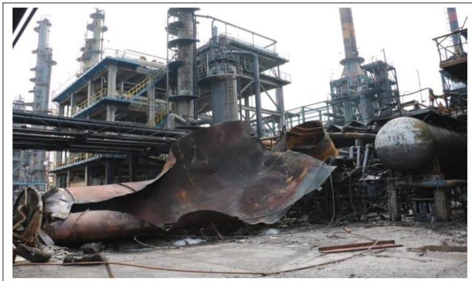
Figure 3: Damaged tank shown in accident scene, ref [1].
