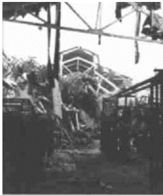
Figure 7 - Scene after the incident (source of the picture: Knowledge Network Node -> link to accident report , retrieved 20.02.2023).
