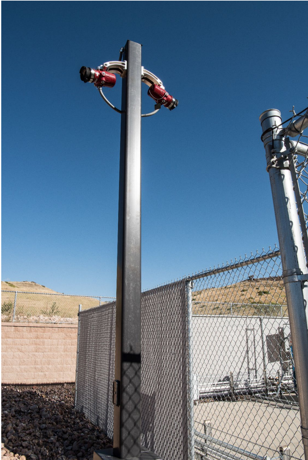
Figure 8. A flame detection system installed at NREL ESIF. Photo by Dennis Schroeder, NREL 40083.
