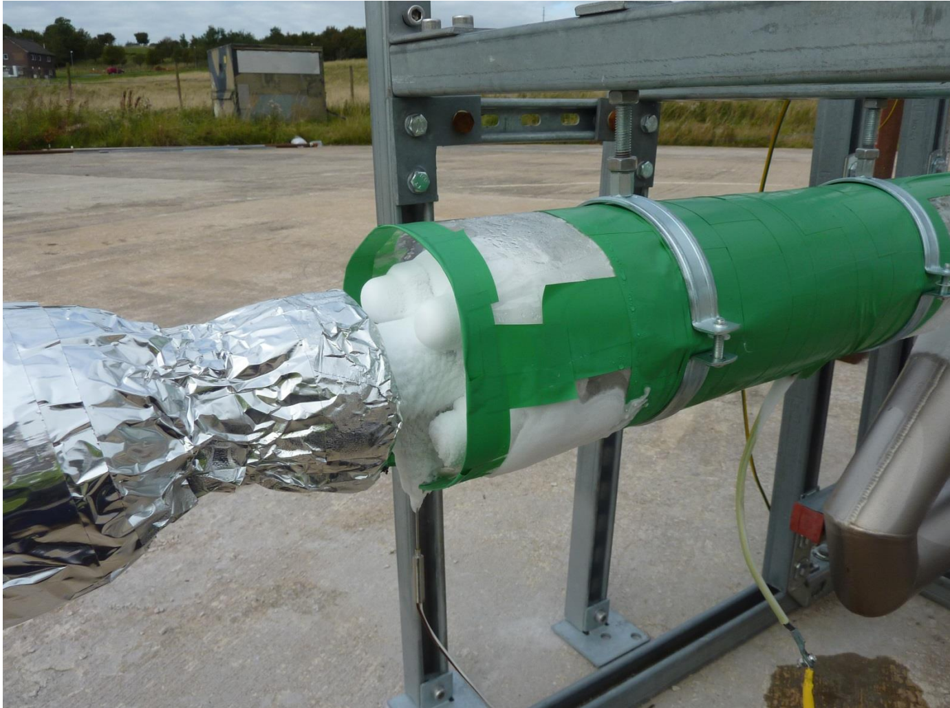
Frost on electrical isolation joint
