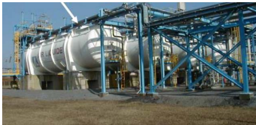
Figure 2-4. LH 2 stores at the Waziers liquefaction plant.
