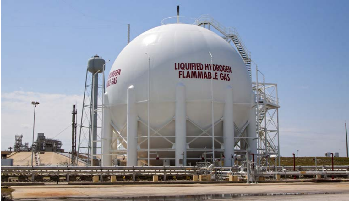
Figure 2-3. LH 2 storage vessel with 3800 m 3 capacity at KSC in Florida (Source NASA).
